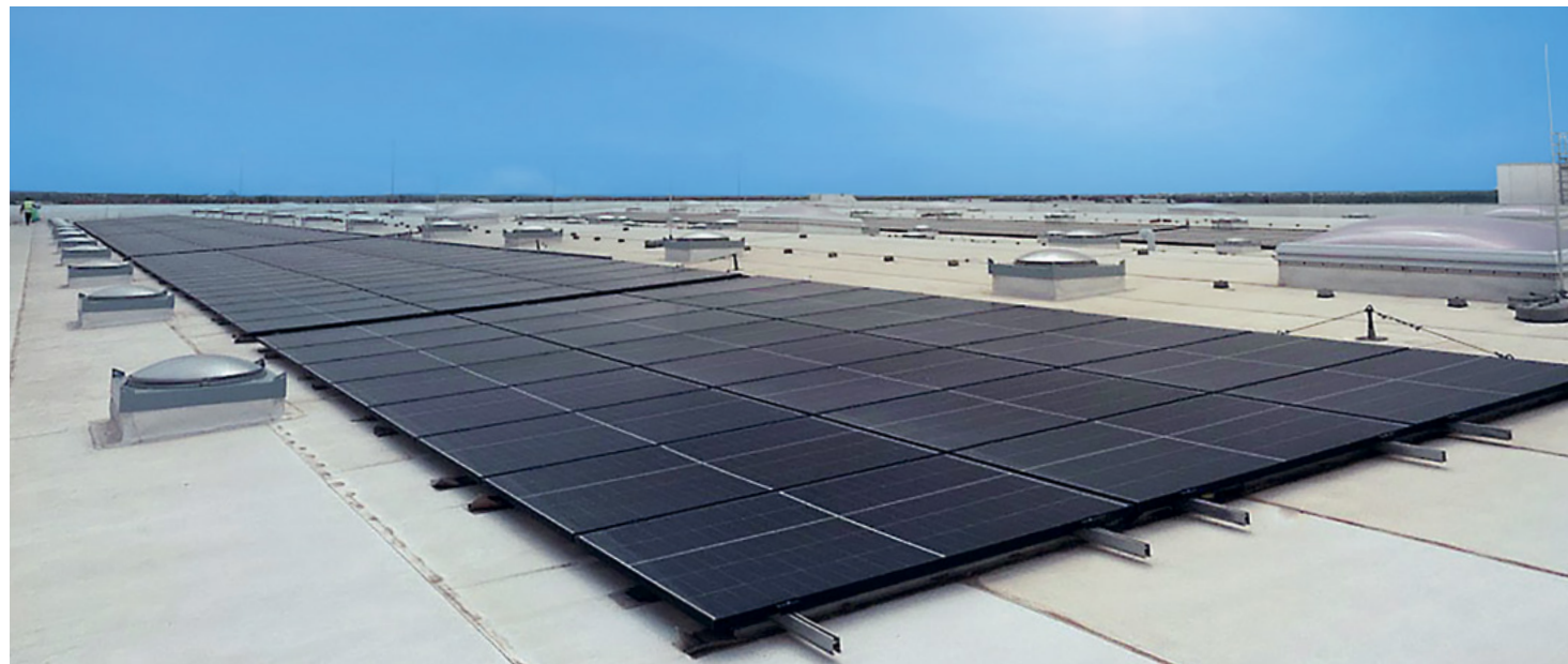
Rooftop photovoltaic system at the production site in Jemmal, Tunisia
