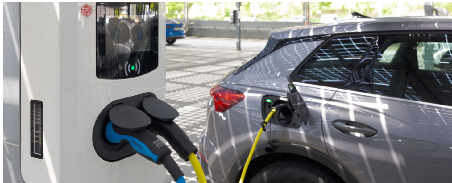
Car park with over 200 charging stations at the main site in Vilsbiburg, Germany
